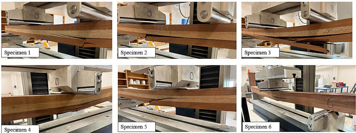
Figure 6. Failure modes of specimens.
