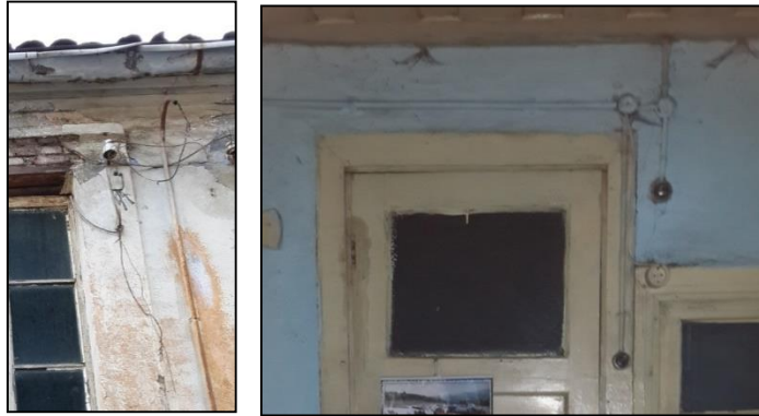
Figure 20. Electrical cables in the building (Created by the author)
