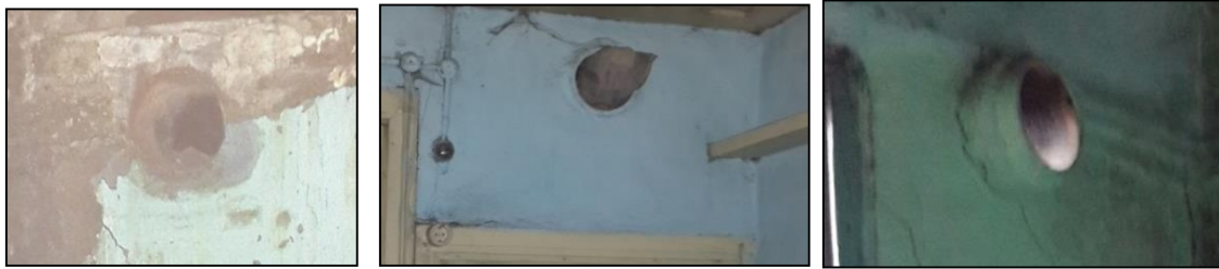
Figure 21. Stove chimney holes drilled later in the building (Created by the author) Figure 21. Stove chimney holes drilled later in the building (Created by the author)
