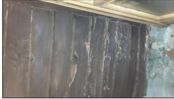
Figure 17. Dampness, rotting and collapse problems on the ceiling (Z-05 living room) (Created by the author)
