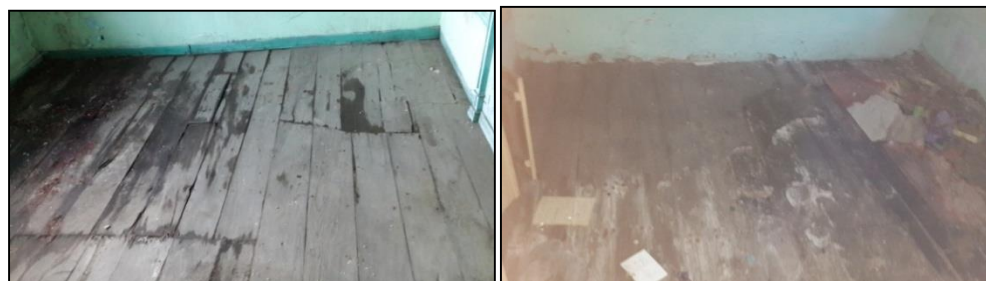
Figure 16. Dampness and rotting problems in the flooring (M-04 and Z-01 floors) (Created by the author)
