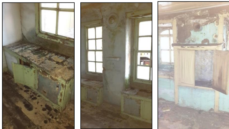
Figure 15. Dampness, moss and rot problems (Created by the author)
