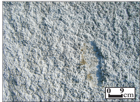
Figure10 - Weak, efflorescence mineralization surface representing gypsum + calcite+bloedite zone.
