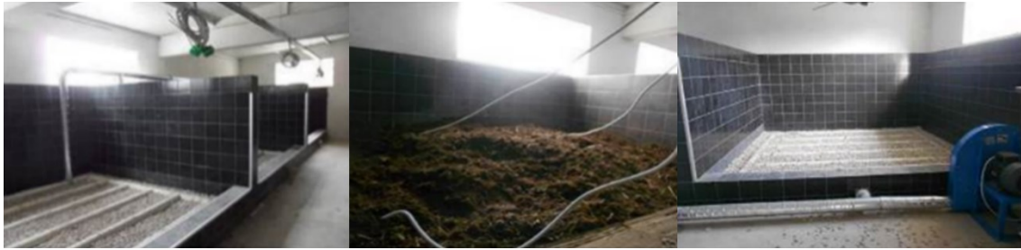
Figure 1. Aerated static pile composting system
