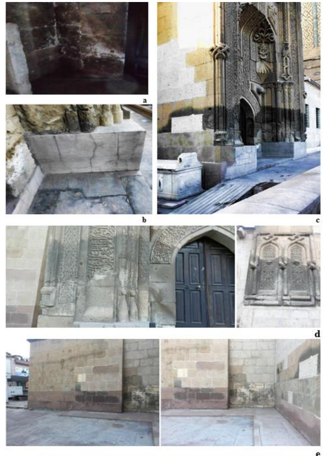
Figure 11. Visibly observed deterioration in the Ince Minareli Madrasa. a- Salt efflorescence on the corridor walls, b- Hairline cracks and surface delamination at the entrance base, c- Rising damp effects on the portal/ taçkapi (author, 2023), d- Surface detachment, and losses in stone carvings observed at the entrance of the portal and at the base of the minaret, e- Discoloration on the exterior walls of the madrasa [61]
