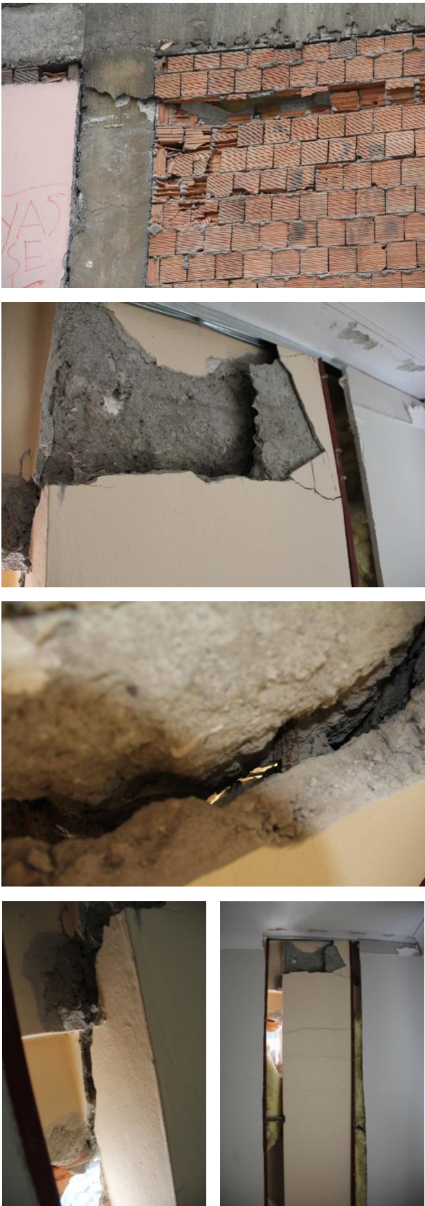
Figure 4. The damaged column (2/2)
