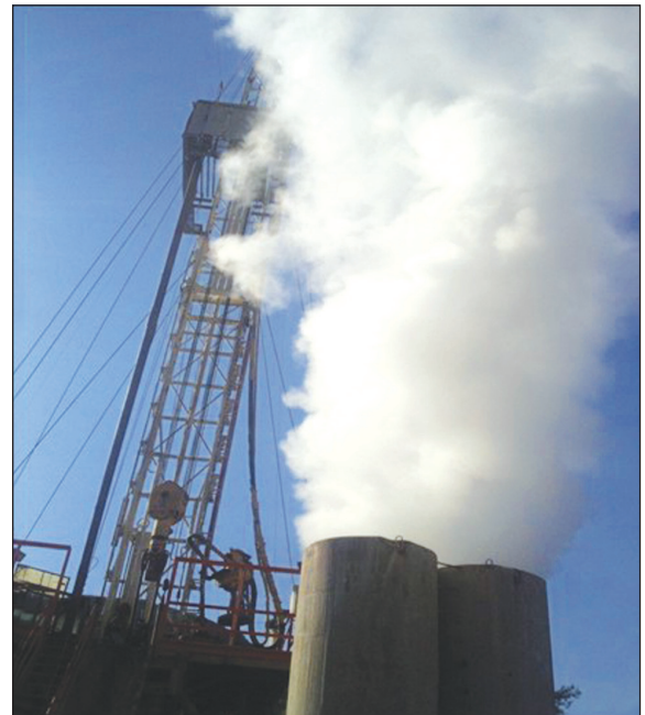
Figure 5- Fluid production in İSA-211/10 geothermal drill.
