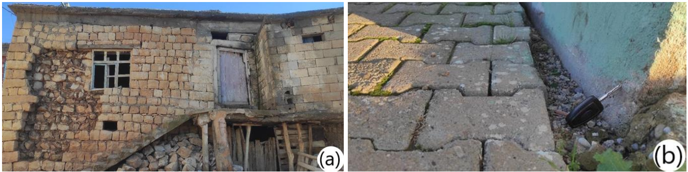
Figure 5. Structural Damage a. Final State of the Structure b. Different Surface Settlement
