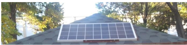
Figure 2. Installed Solar Panel System
