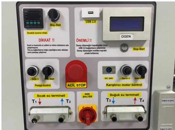
Figure 2 Flow control unit.
