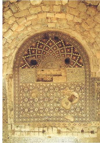
Figure 10 The Church of St. Stephen at Umm al-Rasas (after: Piccirillo 1994: figs. 24-25; courtesy of M. Piccirillo, SBF).
