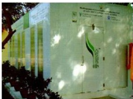
Figure 1. External view of the system (Naik et al. 2014)
