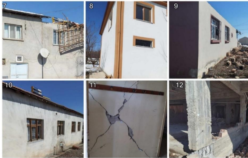
Figure 6: Unchanged Damage Assessment Buildings
