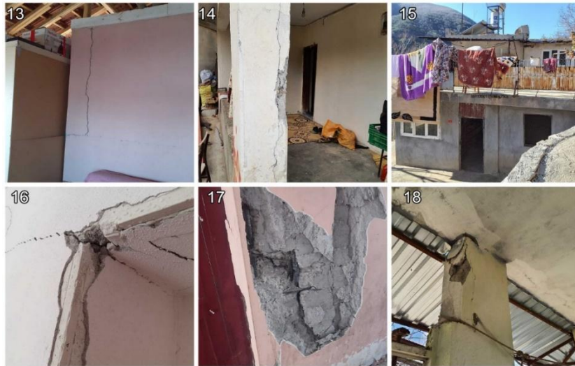
Figure 7: Changed Damage Assessment Buildings
