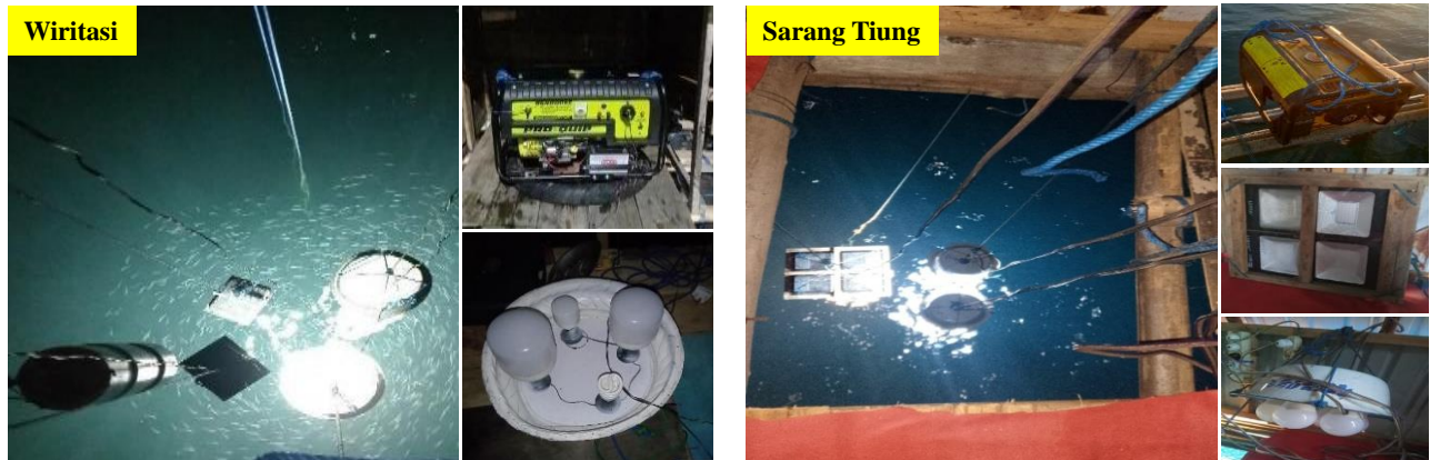
Figure 3. Lighting system performance and portable generators used in study sites
