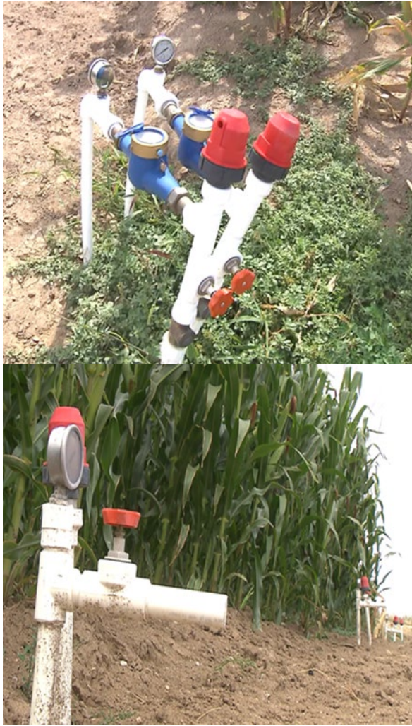
Figure 6. Valves, air-release valves, water meters, and manometers used in SDI.
