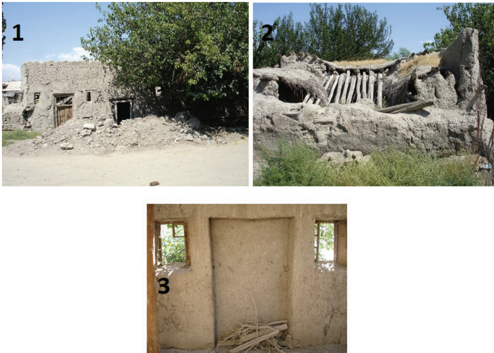
Figure 3. Ruined state of the Kurchulu Mosque; 1-Entrance, 2-Auxiliary building, 3-Mihrab (author's archive).
