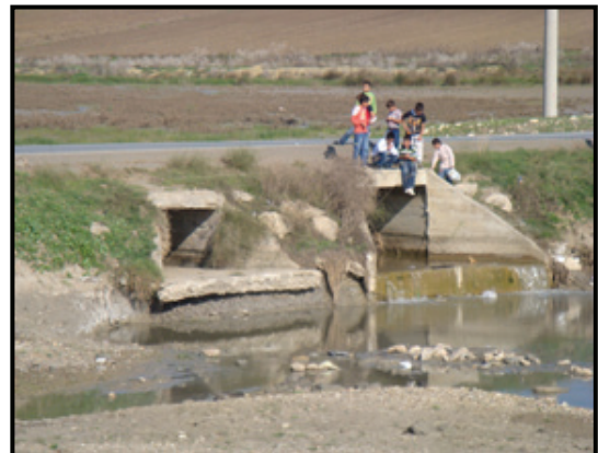
Figure 8. Both pipes and box culverts are insufficient to handle the surface flow.
