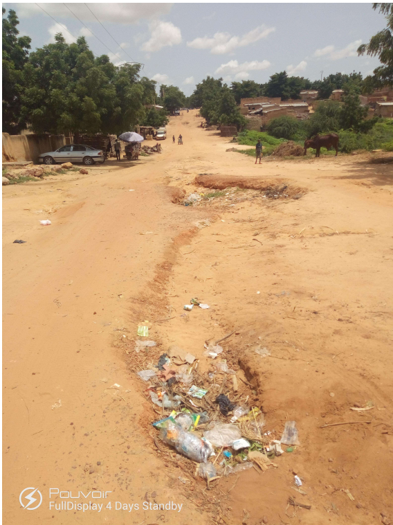
Figure 18: Road Degraded by Gully Erosion source: Abdou Sitou L. (2020).
