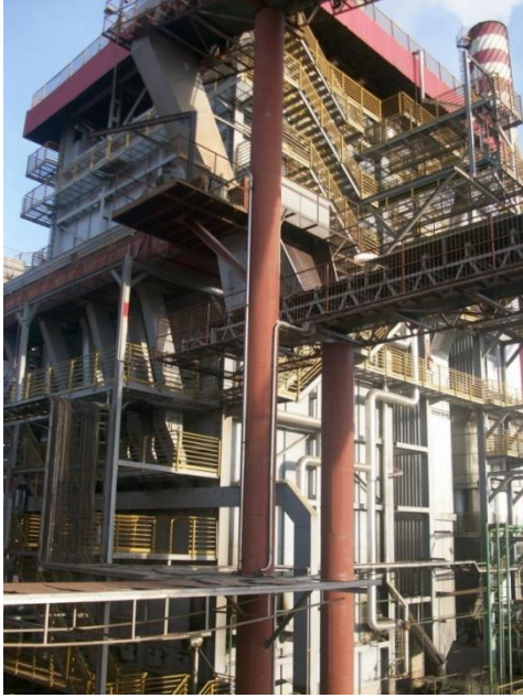
Figure 1b: Bagasse boiler installed in Colombo II mill, (courtesy Equipalcoo Sistemas Ltda).
