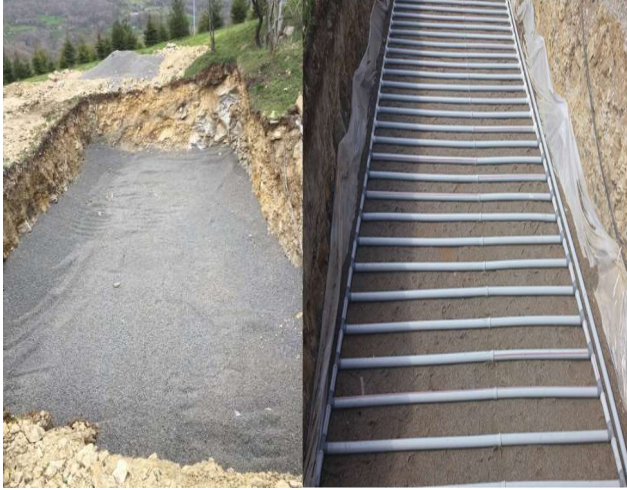
Figure 1. Artificial pond and underground pipe setup [10]
