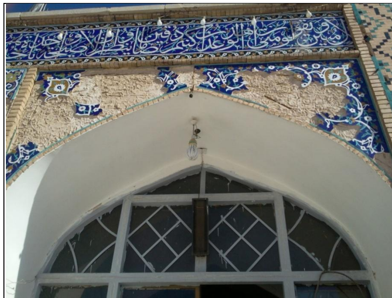
Figure 6. A view of a destruction of the tiles of the interior Sahn of the mosque (Photo: Author)
