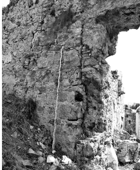
Fig. 7 Sealed door on the western wall of the church (from unit 6a)
