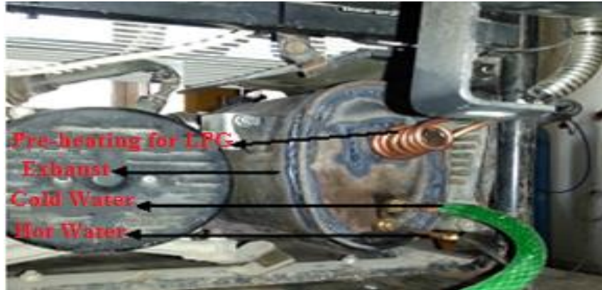
Figure 2. Water connection to the heat exchanger and preheating of the LPG on the exhaust
