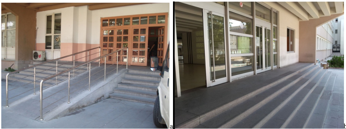
Figure 4 Sec. Building Entrance (to Site Ent-2-Closed CPA) with ramp a:2011, without ramp b:2012
