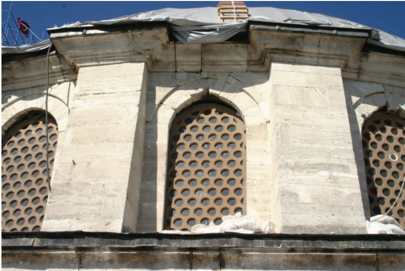
Fig - 4a Damage around station 2 [34].
