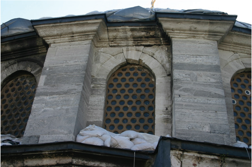
Fig. 8 - Resultant tension cracks around the station 8. Windows were damaged due to tension rod failure causing the dome base to open outwards. Tension rod connection provides horizontal bracing as a diaphragm [34].
