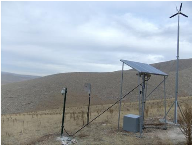
Figure 2. General view of the system on the protection area in Bozdag
