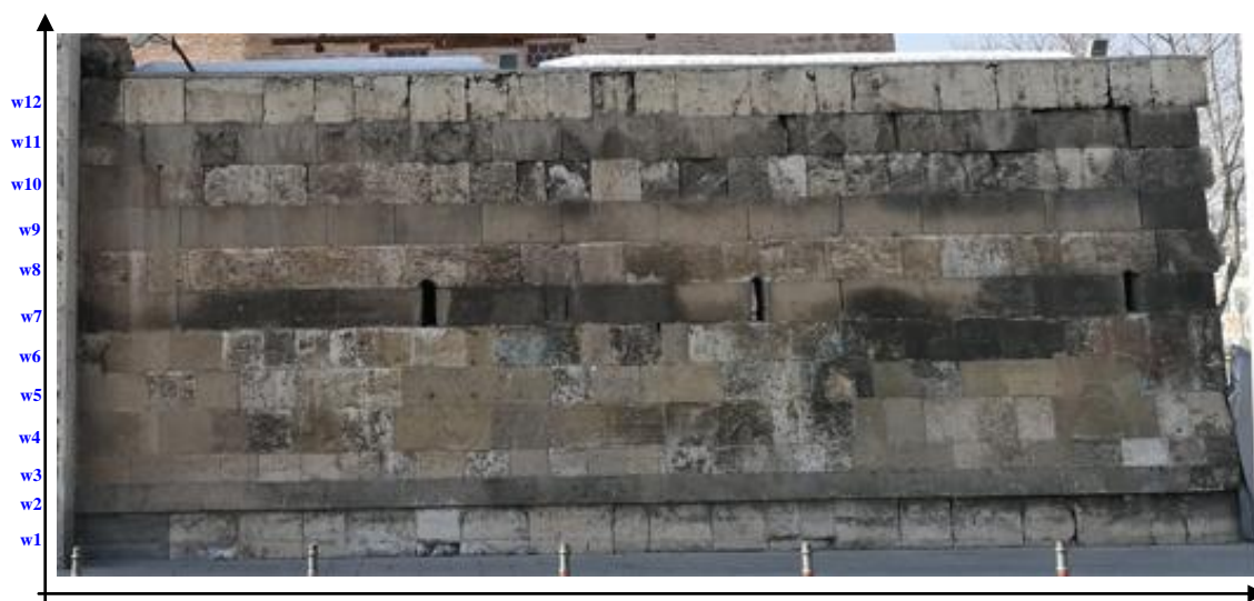
Figure 5. Digitized photograph of Karatay College frontal wall [3]. Dimension stones were numbered according to their positions over the main road (pedestrian, pavement) level.
