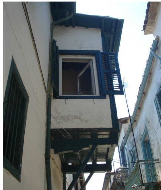
Figure 22- Corbel of Dervish Pasha St. No:15 (Author-2018)
