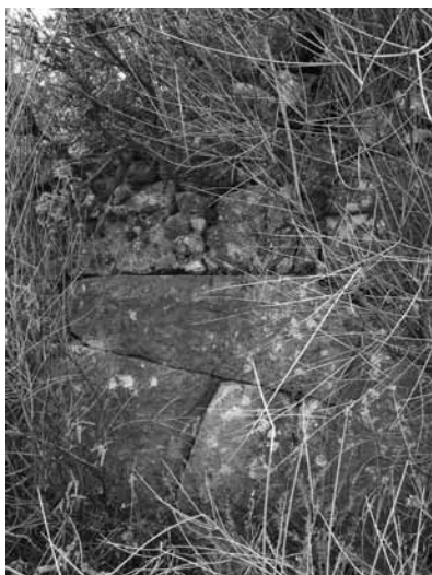
Fig. 6 Haciosmanlar Kayasi, view of the Hellenistic fortification walls with Late Antique repairs
