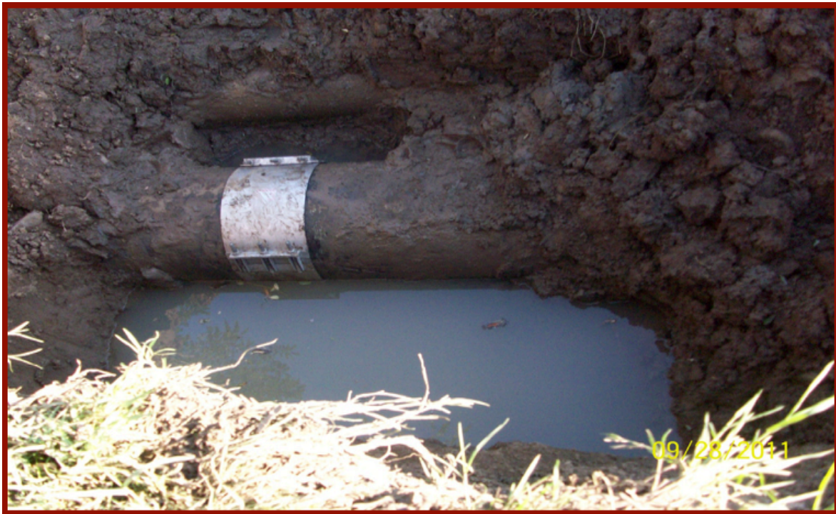
Figure 3. Leaked water from a broken drinking-water pipe was found during the outbreak of Shigella sonnei - Terme City, Turkey, September 2012
