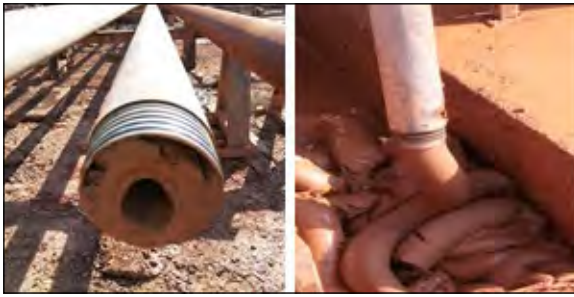
Figure 5- The in-pipe caking and the rate of caking seen during the cleaning of the inside of the pipe.
