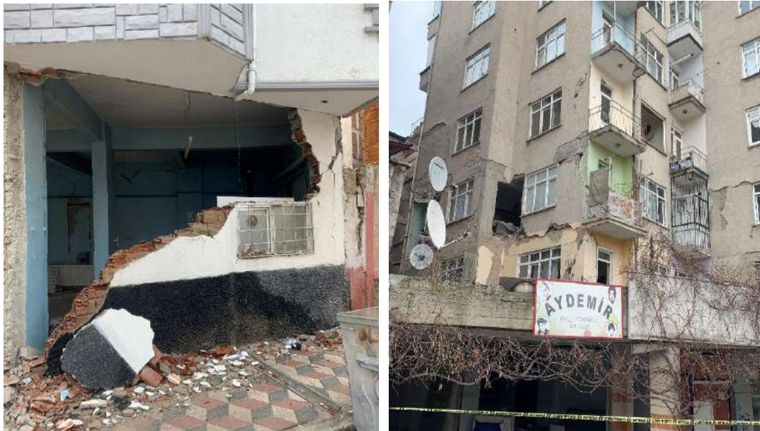
Figure 12 Partial out-of-plane damage
