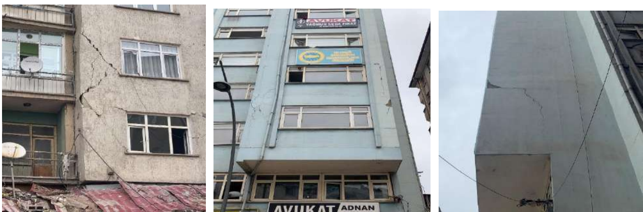
Figure 14 Damages of overhang infill walls
