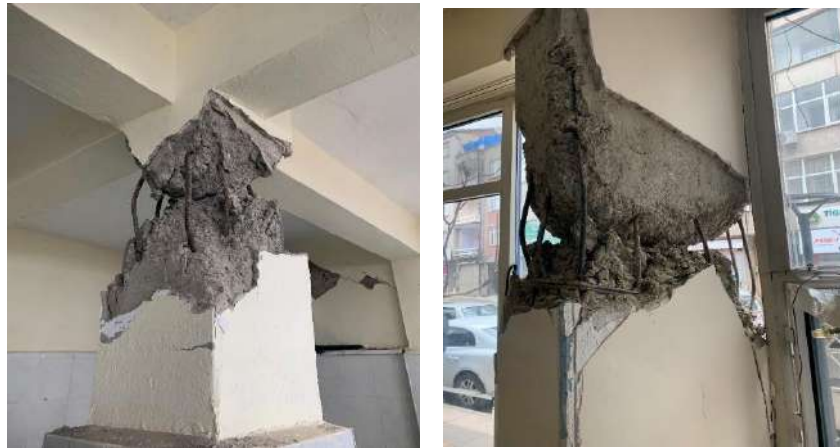
Figure 7 Column damage due to insufficient transverse reinforcement
