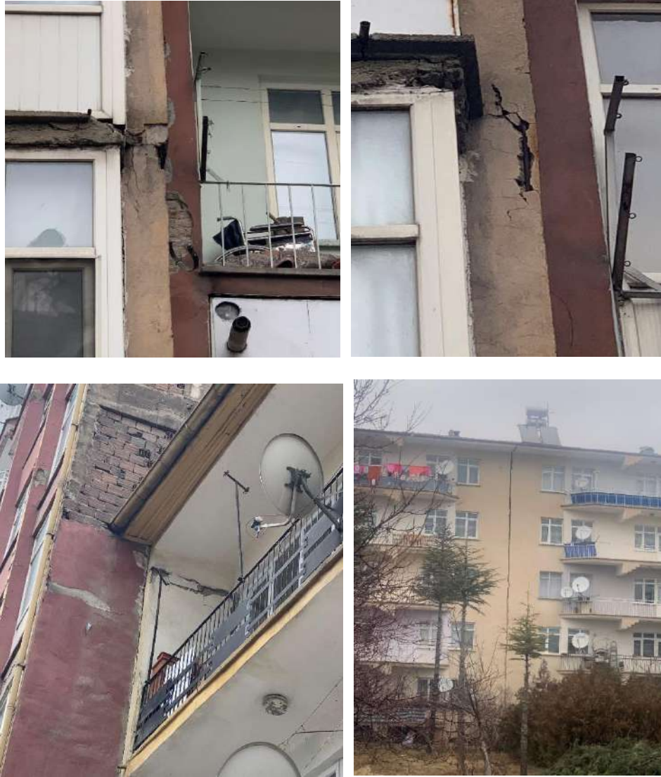
Figure 15 Damages of adjacent buildings
