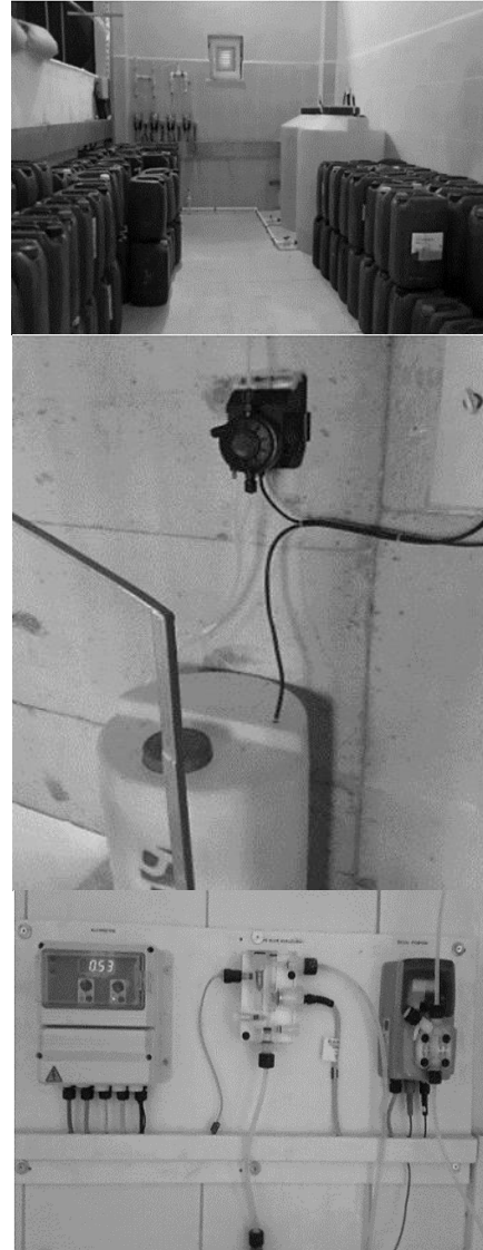
Figure 3. Drinking water sodium hypochlorite system
