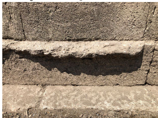
Figure 14 Blockage in front of the stadium
