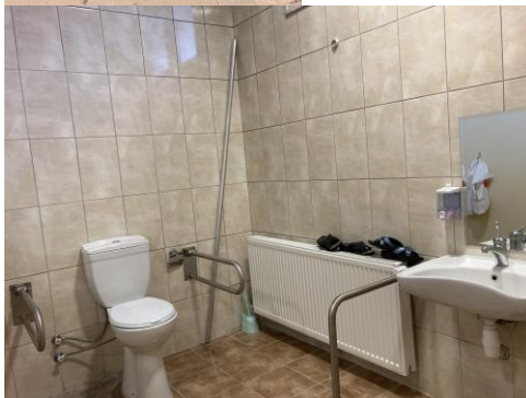
Figure 2-3-4. Faculty of Architecture accessibility arrangements; entrance, interior and WC visuals (Seval Yılmaz, 2022)
