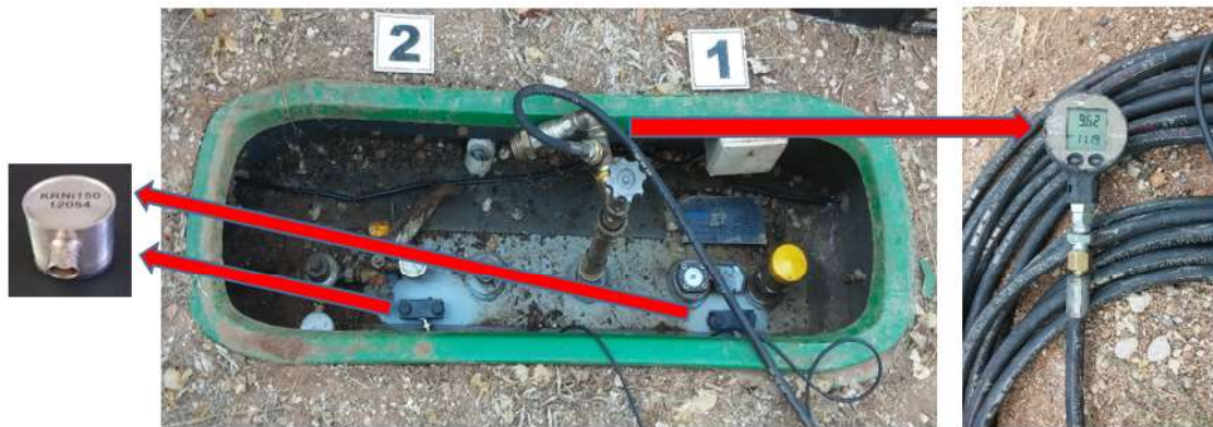
Figure 4: AE sensor mounted on the tank surface and manometer connected to the gas pipeline.
