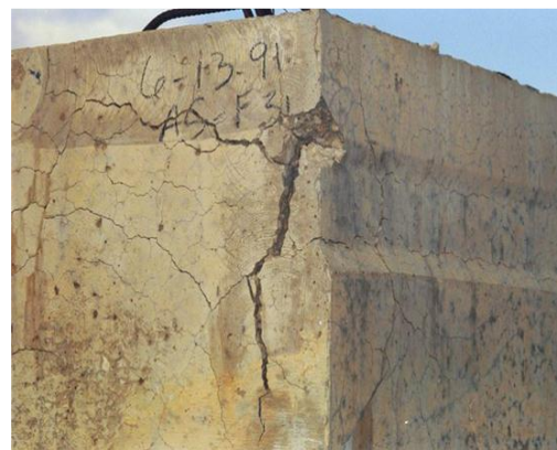
Fig. 2 Micro and macro cracks in a prefabricated beam (Baradan et al., 2013).
