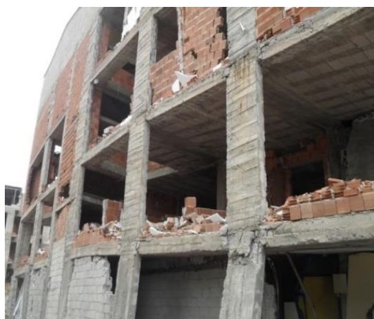
Figure 2. A damaged building with hollow block slab after Van Earthquake (2011)
