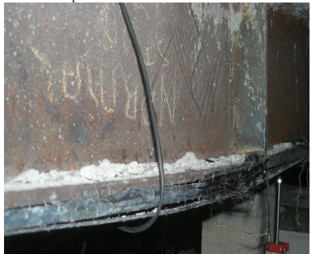
Figure 15. Rupture at edges and de-bonding of CFRP from steel in CBW2CFRP sample
