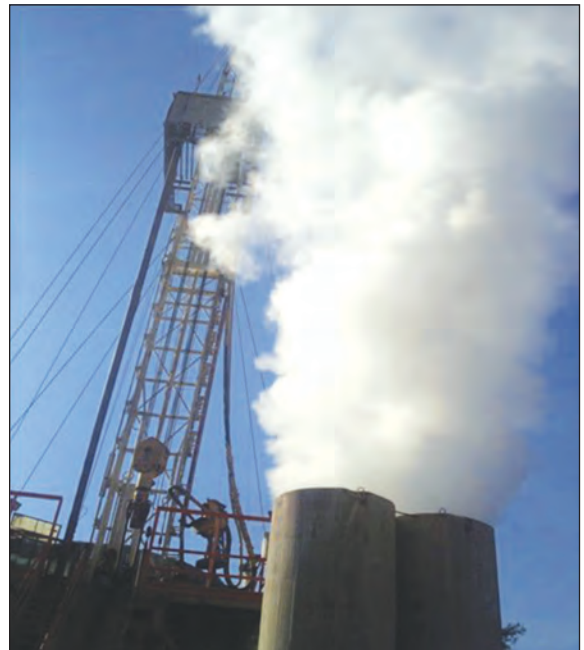
Figure 5- Fluid production in İSA-211/10 geothermal drill.
