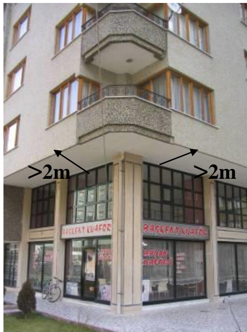
Figure 3. Long, heavy overhangs over a soft storey formation
