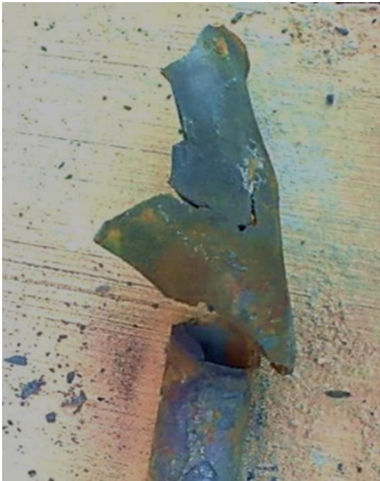
Figure 8. Fracture of a superheater pipe at the knee bends.
