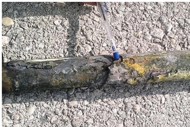
Figure 1. Combustion deposits on the outer surface of the damaged superheater pipe.
