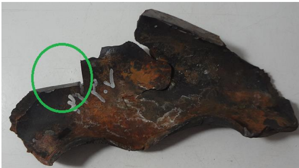
Figure 9. Fracture of a superheater pipe next to the knee bends (Highlighted area is the location used for SEM studies).
