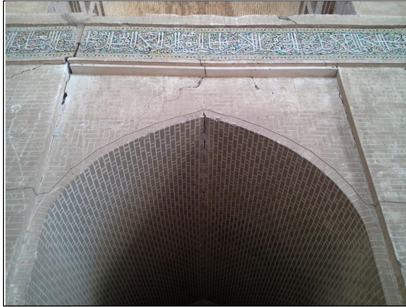
Figure 5. A view of a huge gaps created in the buildings (Photo: Author)
