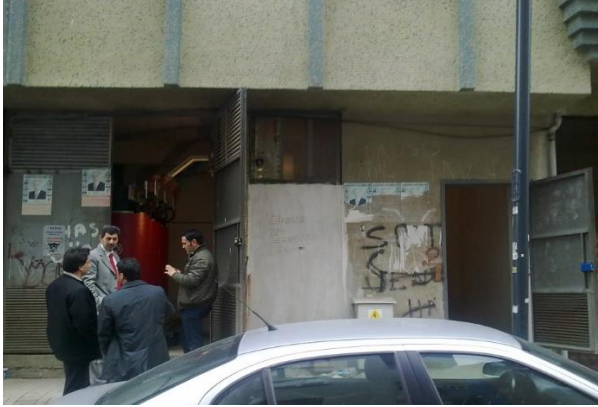
Figure 1. The transformer center from outside
