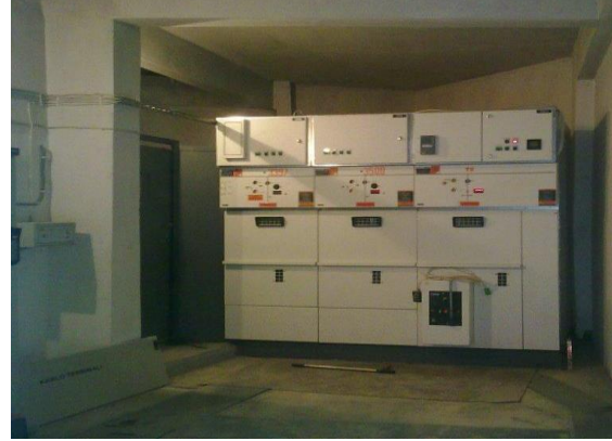
Figure 2. Transformer center from inside -1 (control room)
