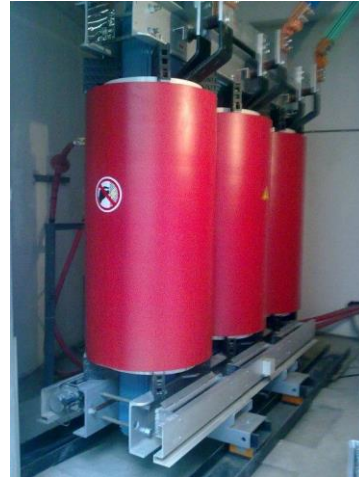
Figure 4. Transformer center from inside -3 (transformer room)
