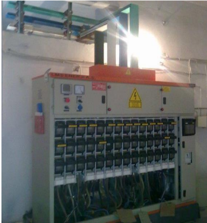
Figure 3. Transformer center from inside -2 (control room)
