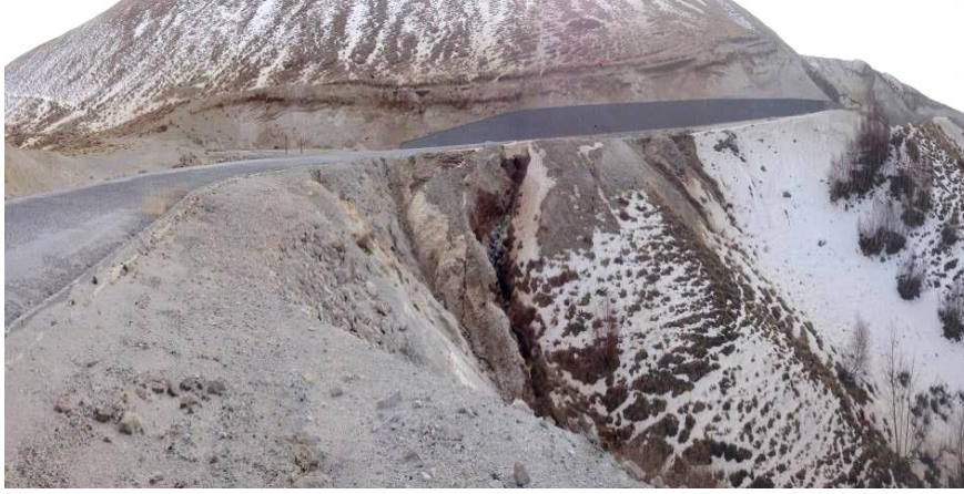
Figure 5. An Image Of The Flows And Slippages Observed In Pyroclastic Rocks At The Entrance Of The Nemrut Caldera Natural Monument (2017)
