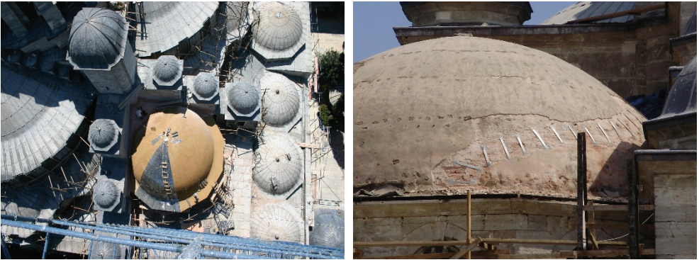
Fig. 6 - Top view from the damaged corner dome next to the main pier station 7 [33, 34]
