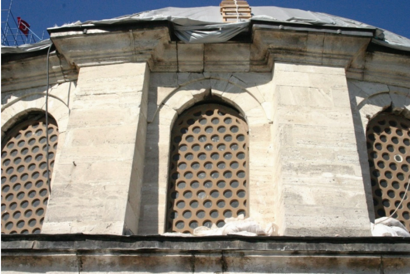
Fig - 4a Damage around station 2 [34].
