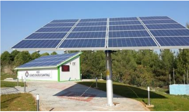
Figure 10. A view of solar PV plant
