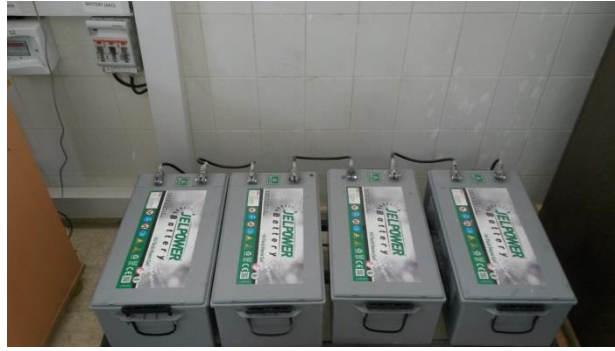
Figure 7. Batteries connected in series with 200 Ah 12 V
