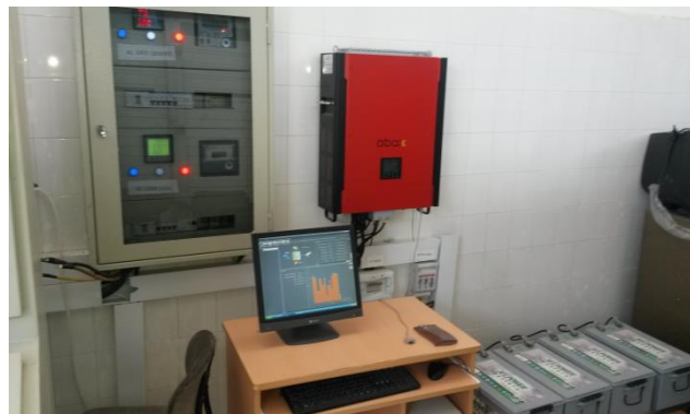
Figure 5. Control and recording system
