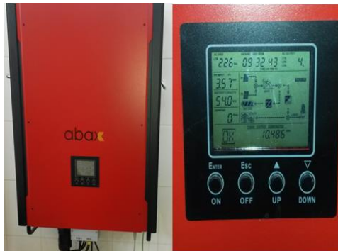
Figure 8. 3 Phase Hybrid Inverter
