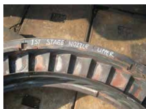
Figure 13. Visual inspection of 1st stage turbine nozzle (erosion material) after operated with B5
