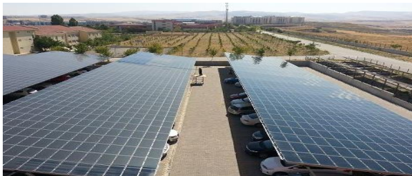
Picture 1: IKCU solar power plant
